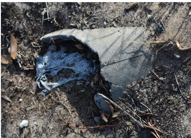
Damaged and blocked drainage
