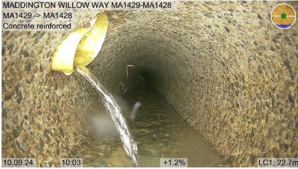
MA1429-MA1428_f1d63ef2-2b51-4b91-94d8-6f753c2a891c_20240910_100308_850.jpg, 00:11:46, 22.70 A connecting conduit is projecting into the conduit being inspected and is obstructing the cross sectional area at 10 o'clock, magnitude of intrusion: 10%
