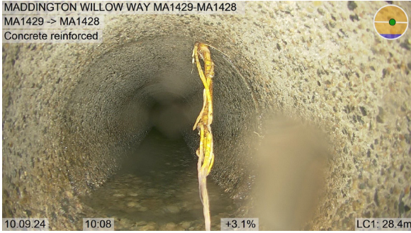
MA1429-MA1428_f41b46cf-80de-45af-8aa8-25456dc3bfc2_2 0240910_100814_200.jpg, 00:14:52, 28.40 Tap roots, reduction in cross sectional area, Obstruction: 10%, at joint at 1 o'clock
