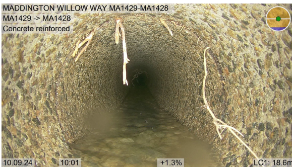
MA1429-MA1428_53558f7d-7d27-49e3-99e6-1b59f5815b5f_2_0240910_100113_097.jpg, 00:10:31, 18.60 Recently cut fine roots-a relatively small number of cut minor roots remain, Obstruction: 10%, at joint from 10 o'clock to 2 o'clock
