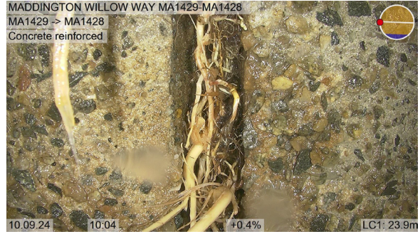
MA1429-MA1428_e0912fb9-4600-429c-af7e-9c2cccd9786a_20240910_100449_386.jpg, 00:13:12, 23.90 Recently cut interwoven mass of mostly fine roots leaving a beard of roots, Obstruction: 10%, at joint from 8 o'clock to 5 o'clock
