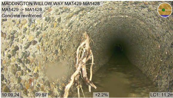
MA1429-MA1428_a05fe89a-3092-4720-a548-5f72f5b2b79f_2_0240910_095715_589.jpg, 00:07:01, 11.20 Recently cut tap roots, a small number of cut major roots (10mm or greater) is evident, Obstruction: 20%, at joint from 7 o'clock to 10 o'clock
