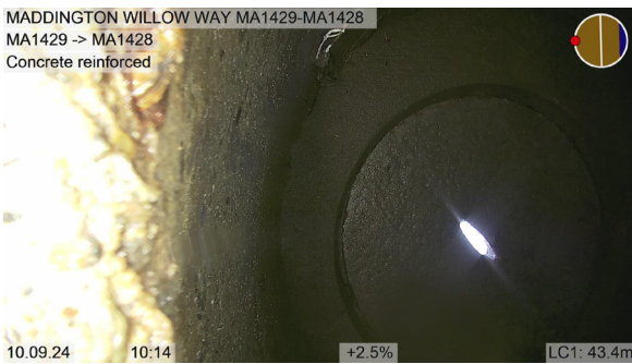
MA1429-MA1428_da65eb16-e39b-435d-a734-6d1ae6917588 _20240910_101432_836.jpg, 00:20:31, 43.40 Surface damage concrete, spalling of the concrete conduit including localised chipping from 12 o'clock to 12 o'clock, Finish
