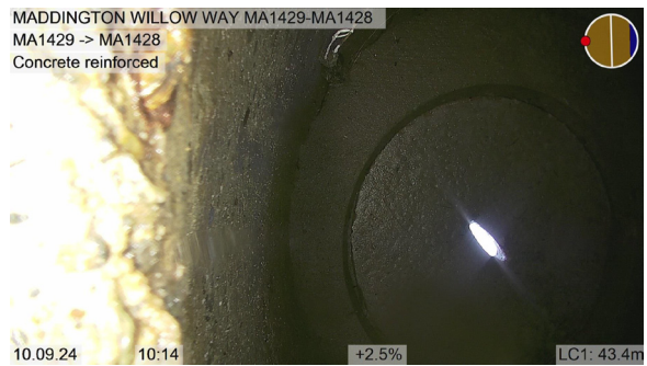
MA1429-MA1428_3002bd45-befa-4c54-b667-4618f866f53c_2 0240910_101451_674.jpg, 00:20:38, 43.40 Finish node, maintenance chamber, Nodename:, MA1428
