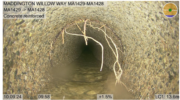
MA1429-MA1428_6f346f7b-4b3d-4e14-b05a-f59bc15156c7_2_0240910_095859_550.jpg, 00:08:31, 13.60 Recently cut fine roots-a relatively small number of cut minor roots remain, Obstruction: 10%, at joint from 10 o'clock to 2 o'clock
