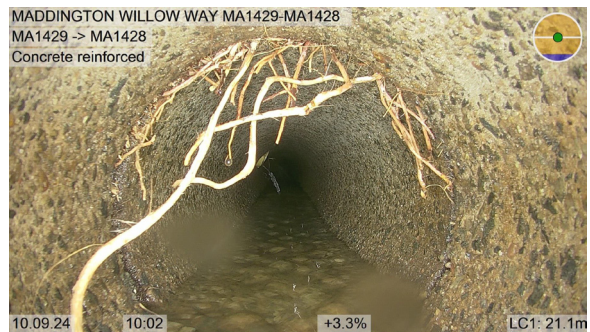
MA1429-MA1428_36046084-1a0b-47c0-932c-a0a5ad31acae_20240910_100215_836.jpg, 00:11:12, 21.10 Recently cut interwoven mass of mostly fine roots leaving a beard of roots, Obstruction: 20%, at joint from 9 o'clock to 3 o'clock
