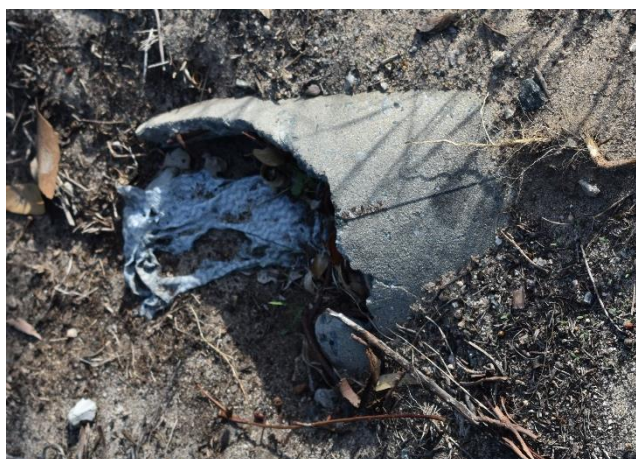
Damaged and blocked drainage
