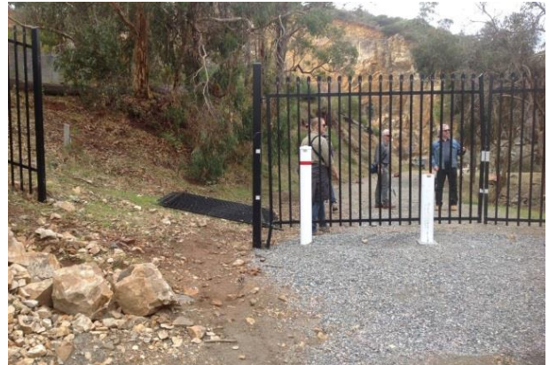
Plate 25: Broken Gates leading to Barrington Quarry
